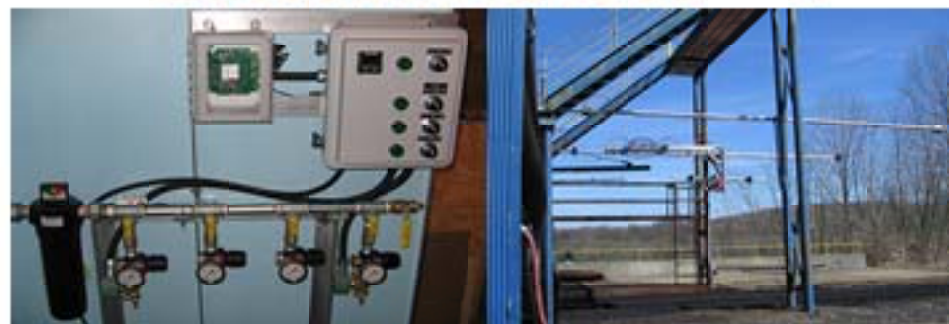
Railcar Spray System
